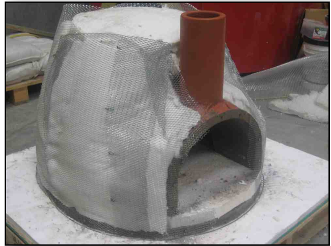
7.2. Stucco lathe holds the FB Board in place and can shape the Igloo.
